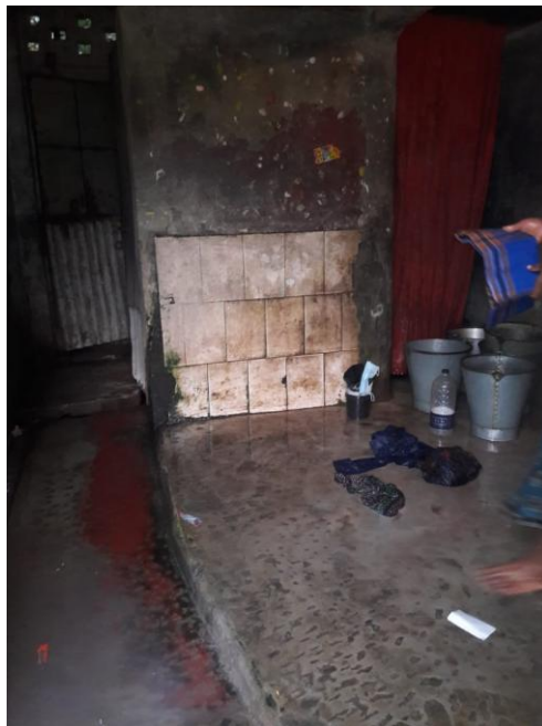
Plate 12. Photograph of water source of the slum dwellers (III)
