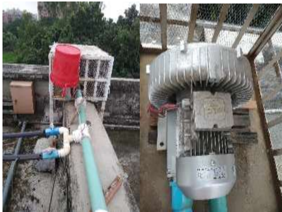
Bubbling and pumping system
